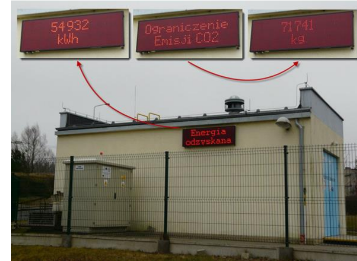
Testing of energy storage concepts integrated into trolley grid / substations (incl. 2 nd life batteries) (TU Delft, PRE, Szeged)
